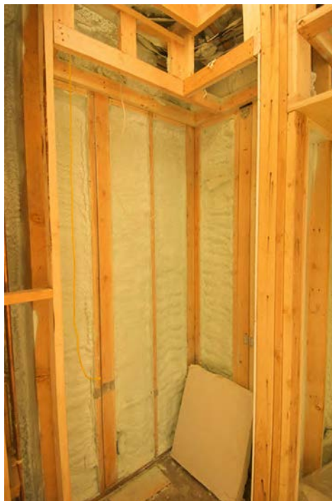
Figure 1.20 Insulation is used to limit the conduction of heat from the inside to the outside (in winter) and from the outside to the inside (in summer). (credit: Giles Douglas)
