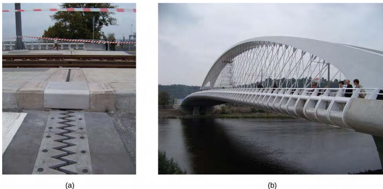
Figure 1.5 (a) Thermal expansion joints like these in the (b) Auckland Harbour Bridge in New Zealand allow bridges to change length without buckling. (credit: “ŠJů”/Wikimedia Commons)
