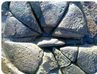
Figure 112: Stress caused these rocks to fracture.
