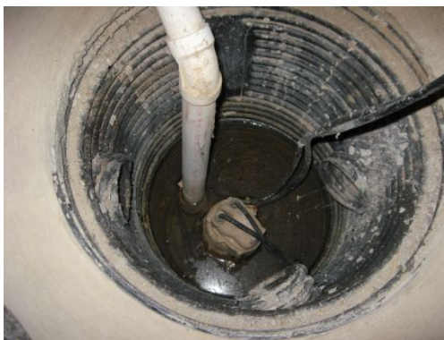
Figure 6.4.2: A sump crock.
