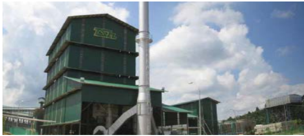
Figure 45: Janal Landfillbiogas power plant.
