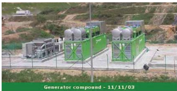
Figure 44: THS bioenergy plant.
