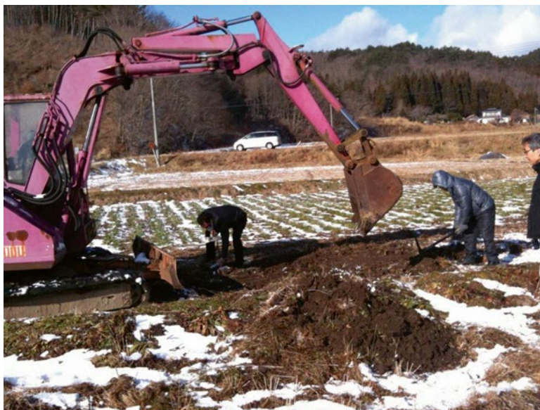
Fig. 13.5 Stripping the frozen soil using a backhoe by a local farmer on January 8th, 2012
