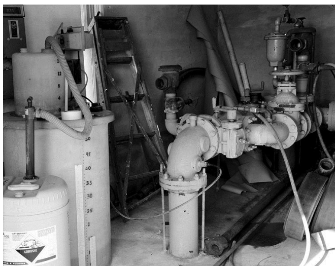
Figure 5-1 Feed pump application of fluoride compound into drinking water – Image by the Library of Congress is in the public domain
