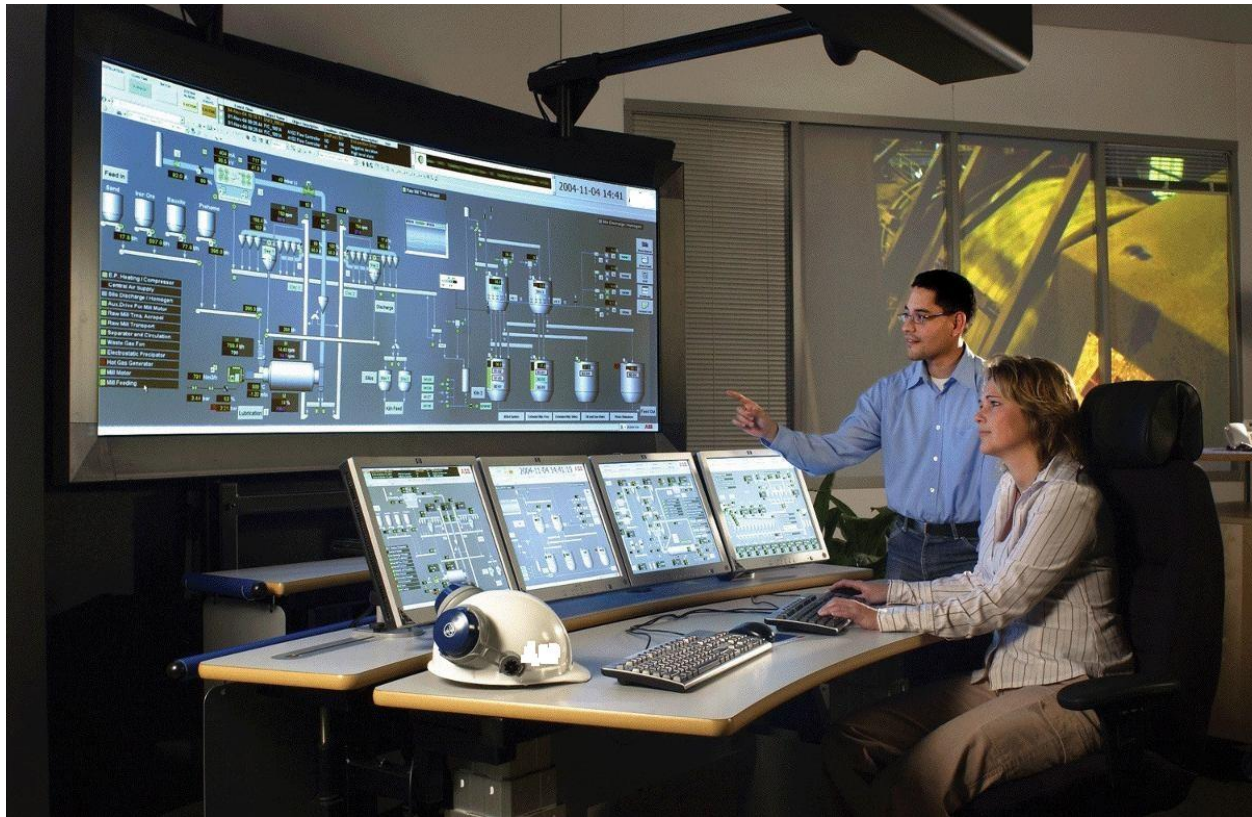
Figure 11-2 SCADA Control Monitor – Image by hhdgomez is licensed under CC BY-SA 4.0
