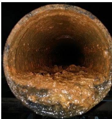
Figure 6-2 Corrosion in pipe with tubercle buildup – Image by Mr pantswearer is licensed under CC BY-SA 3.0
