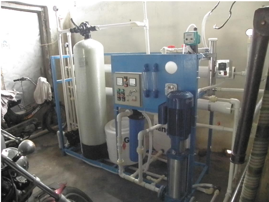
Figure 10-4 RO Water Treatment – Image by Vishalsh521 is licensed under CC BY-SA 3.0
