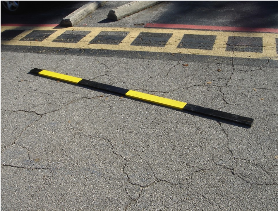
Image 15.1 – Broken Parking Lot Board
